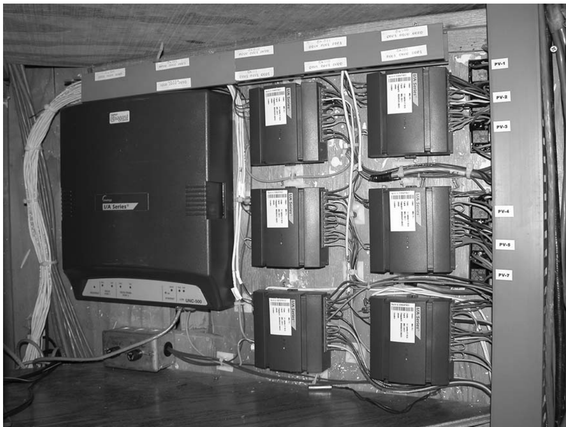
Figure 7.11 Photograph showing control closet hardware.
