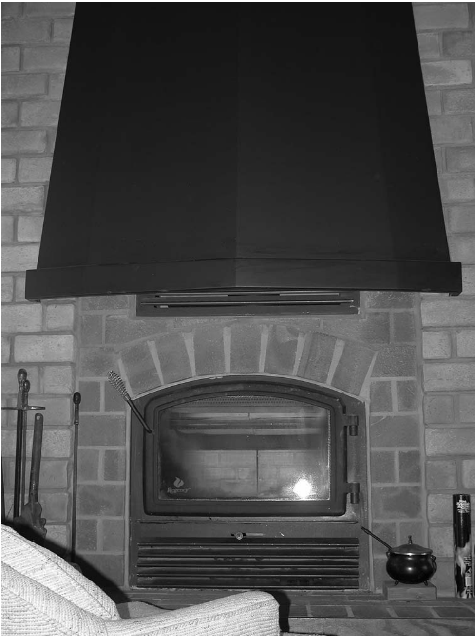
Figure 7.12 Photograph showing heat-producing fireplace.
