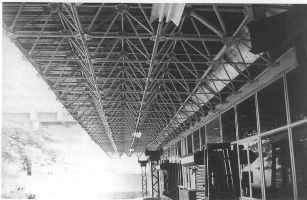
Fig. 1.4. The space frame over the arrival hall at Bangalore Airport, Bangalore, India
