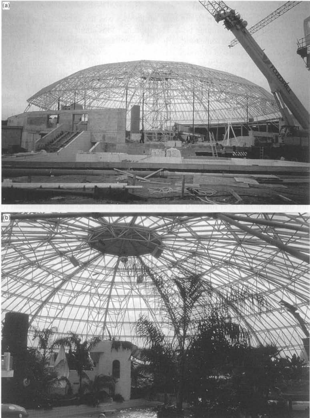
Fig. 8.23. The Aquadrom, Bremen, Germany: (a) the dome near completion; (b) the finished dome
