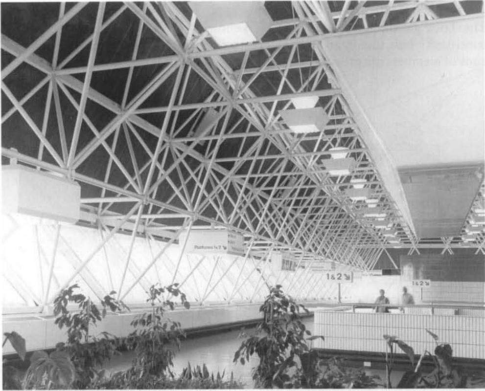
Fig. 1.8. The Nodus space frame over the concourse of the Gatwick railway station
