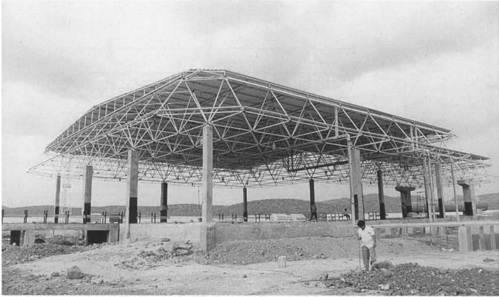
Fig. 1.14. The space frame over the domestic cooking gas bottling plant, for the Indian Oil Corporation, Cuddapah, India
